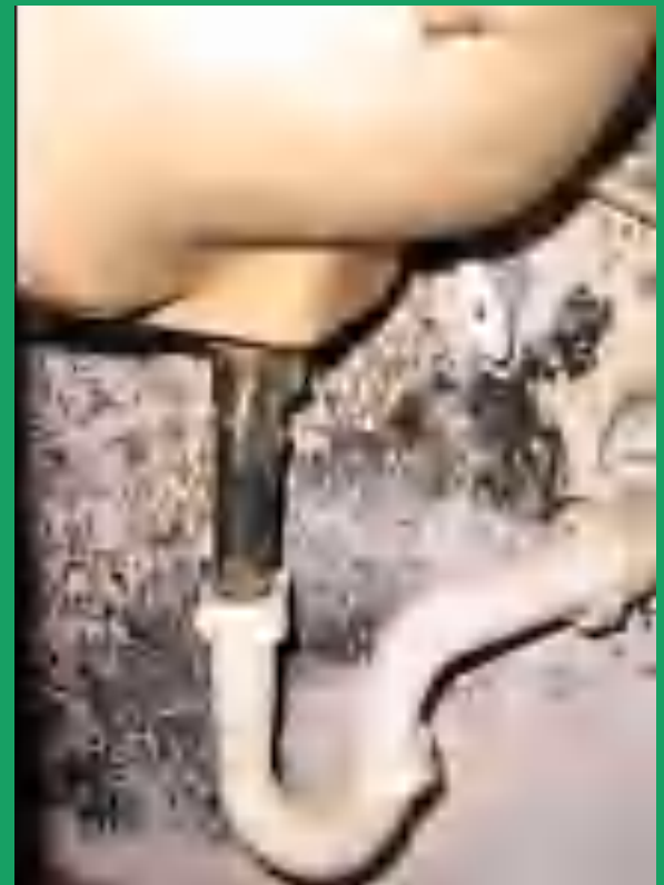
Mold growth under a leaky sink
